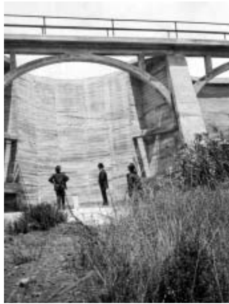
Downstream face of Murray Dam, 1917, showing one arch of the multiple arch structure. Courtesy of the Helix Water District Archives.
